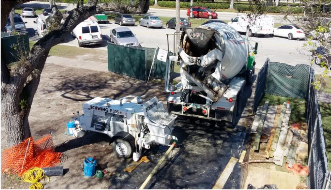
The newly poured roof over what will be the school and business entrance.
