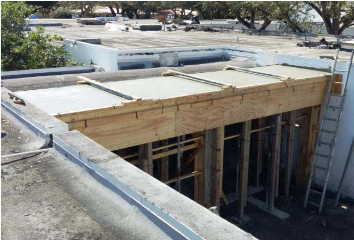
The base layer of Poured in Place outdoor play surface going on.
